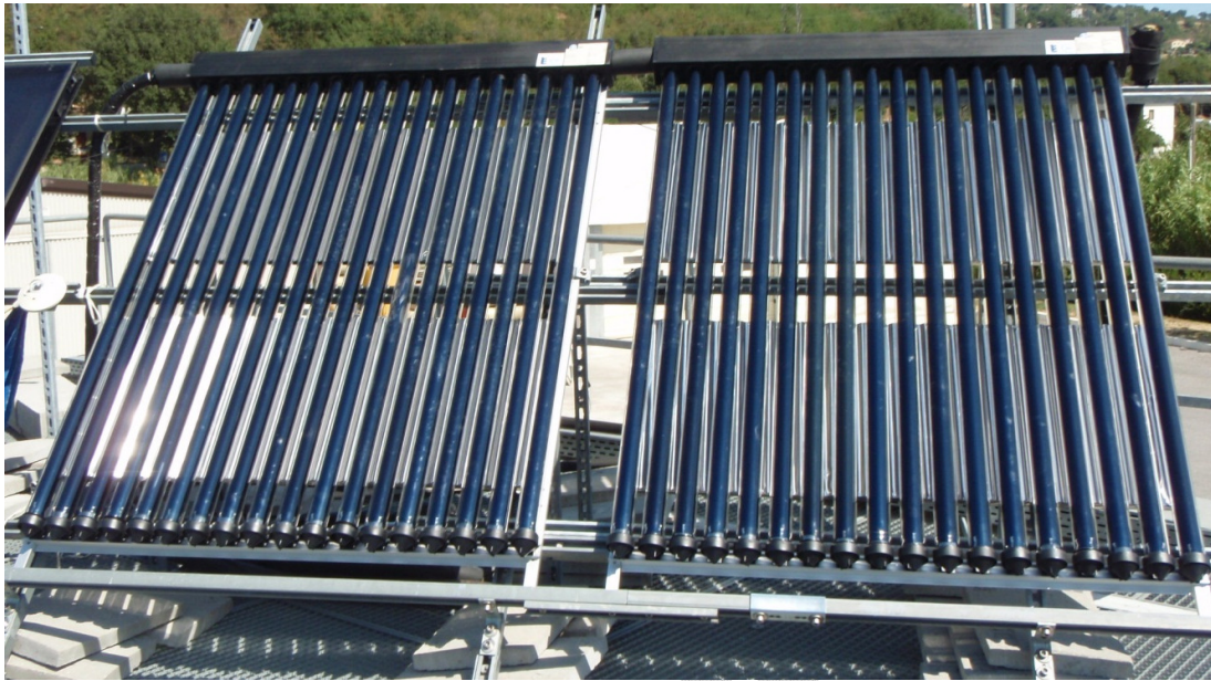
Fig. 1: Evacuated tube collector area
